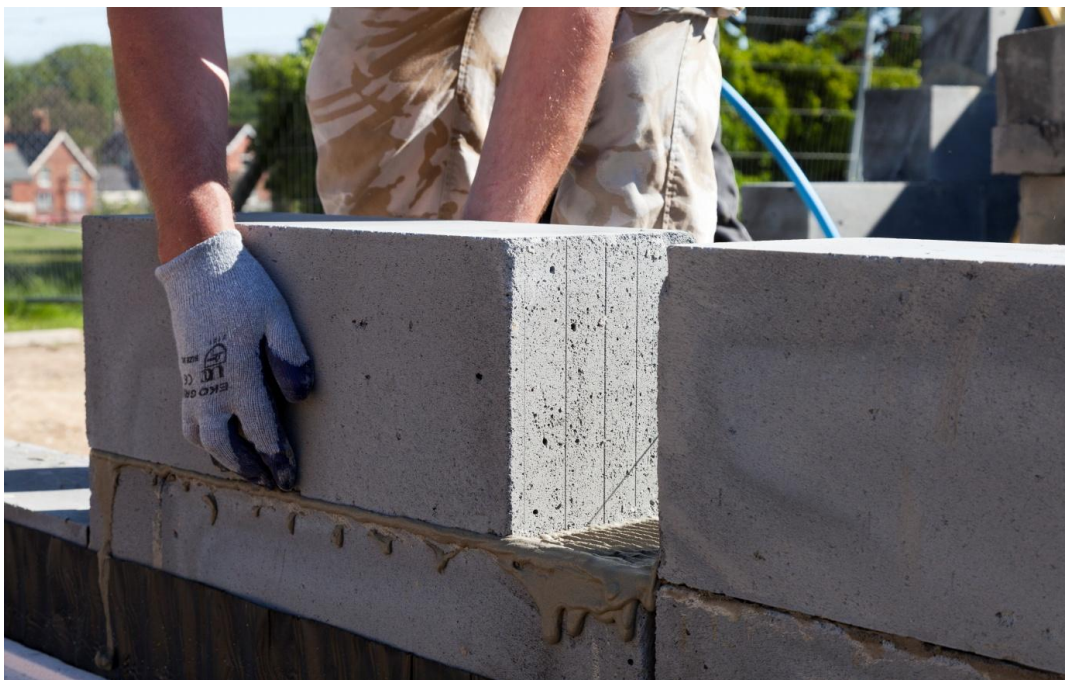
Fly ash has a variety of applications including durable concrete blocks for house building
