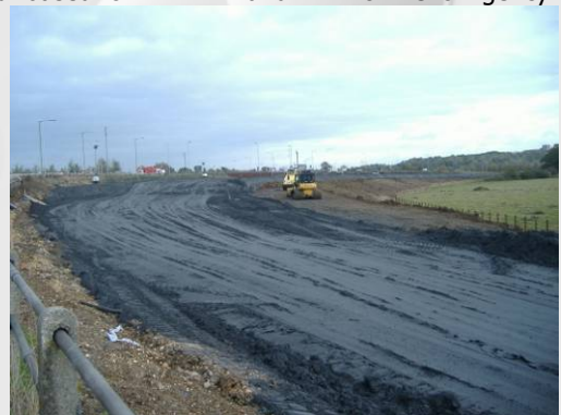
Figure 1 - A new slip road from the A4211 to the M1 using PFA for the embankment
