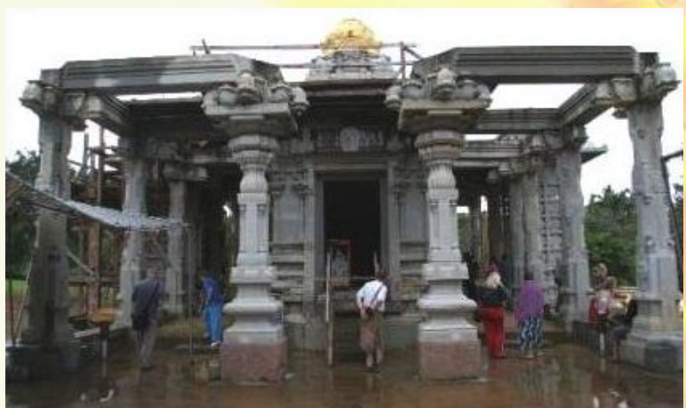
Figure 2 – HVFA was used for a massive, monolithic foundation slab at the Hindu Temple, Kauai Island, Hawaii, 1999
