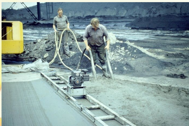
Figure 1 - HFCC laid at Didcot Power Station in 1981 Apologies for lack of Health and Safety equipment
