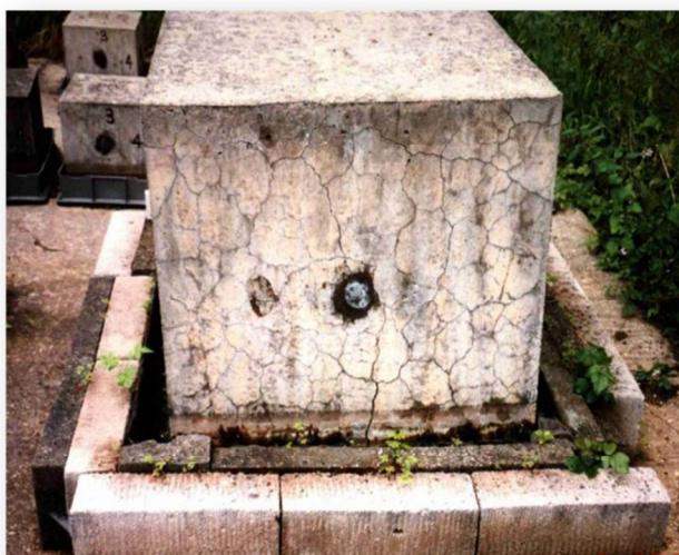
Figure 1 - ASR in PC concrete
