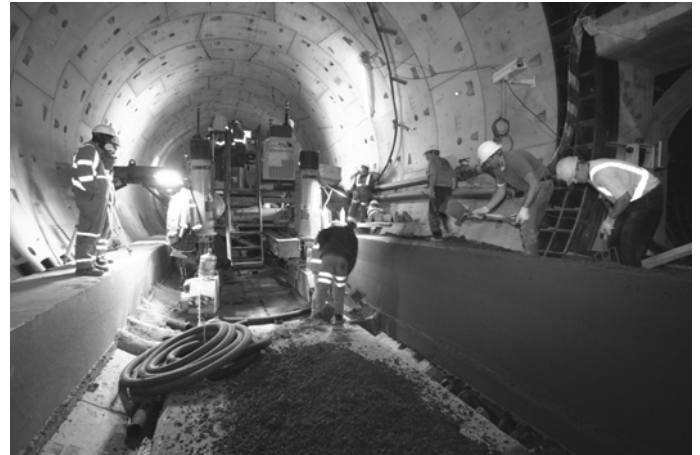
Figure 2. Channel Tunnel Rail Link used PFA to reduce thermal cracking and enhance durability.
