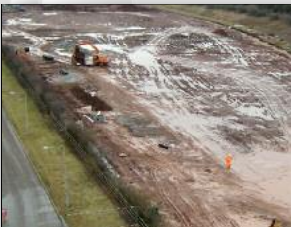
Figure 2 - The site prior to any treatment, when only the topsoil had been stripped and the ground was being prepared for the fly ash lime operation. As will be seen it was a rather wet time of the year
