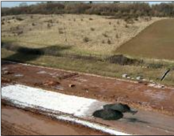
Figure 4 - shows an area of fly ash being treated with lime immediately prior to rotovation
