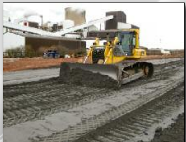
Figure 3 - Shows the fly ash being levelled after lime has been spread and rotovated into the fly ash. This is then trimmed to level
