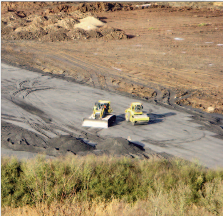
Figure 2 - The PFA was bladed out at 200mm thickness and then compacted to 150mm
