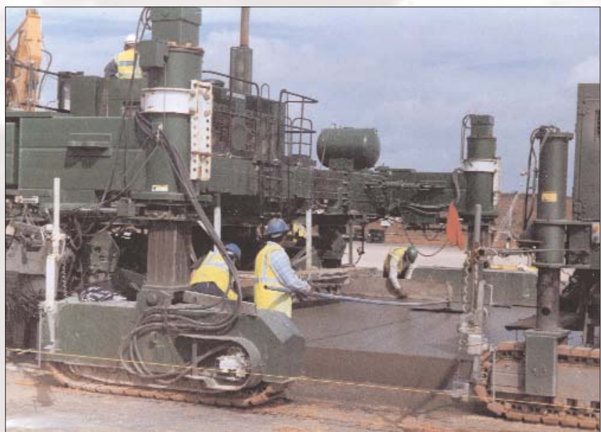
Fly ash concrete being used on East Midlands Airport taxiways (courtesy of Fitzpatrick Contracting Ltd)
